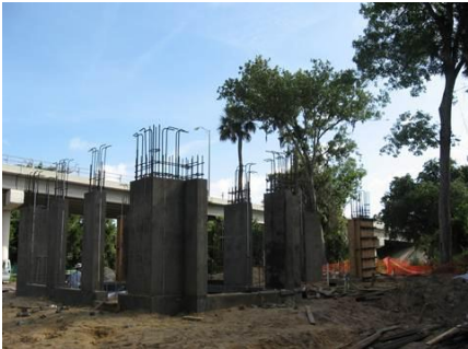
Pump Station Generator Building
