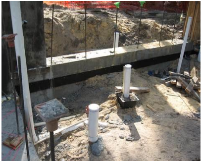
Generator Building Plumbing
