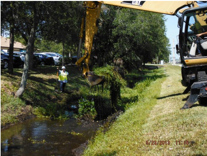
Cleared 3.168 linear feet of weed mat from ditch on Palm Coast Parkway
