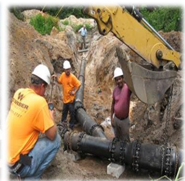
12" Ductile Pipe to Manhole
