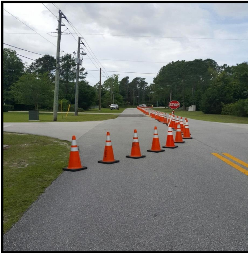
Setting up MOT for asphalt repair at Bird of Paradise Drive & Birchwood Drive
